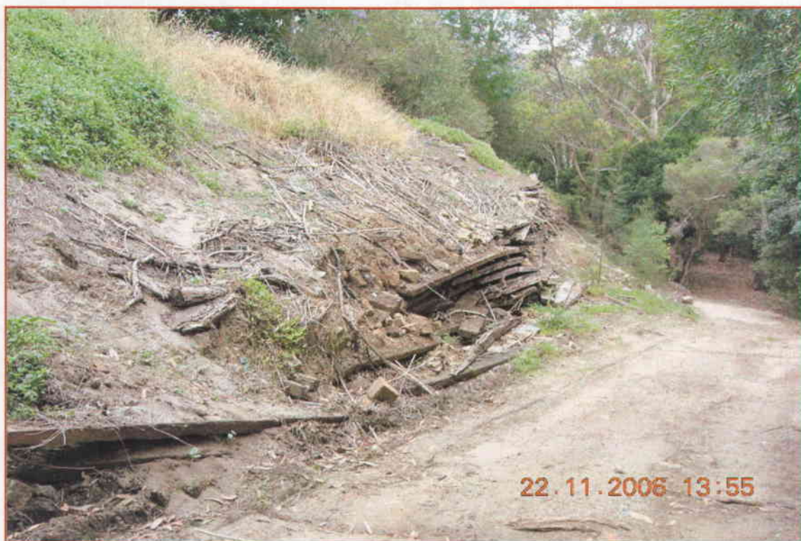
PHOTO 10: Failed crib wall
