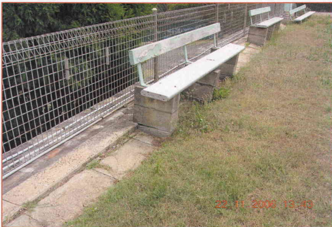
PHOTO 6: Settlement of filling
